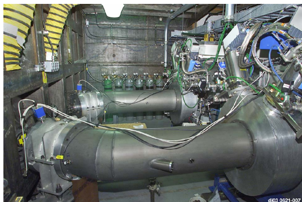
Figure 3. Cygnus installation at the U1a Complex. Top - Marx generators, Middle - Stalks removed from IVAs, and Bottom - VITLs (center) and angled Diodes (far left).
